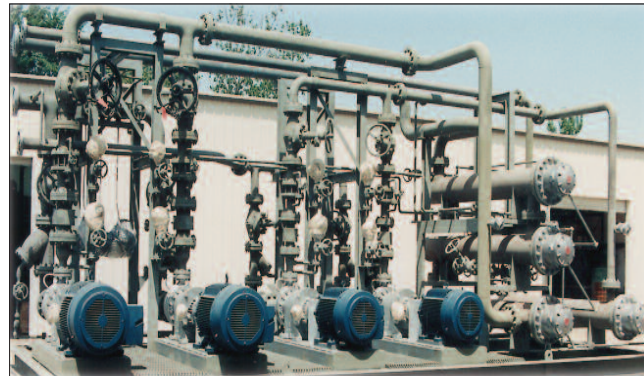
Dual zone, mag drive pump for petrochemical
