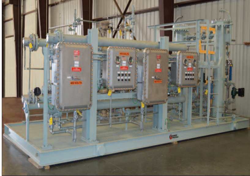
Redundant NEMA 7 panels for un-manned compressor station
