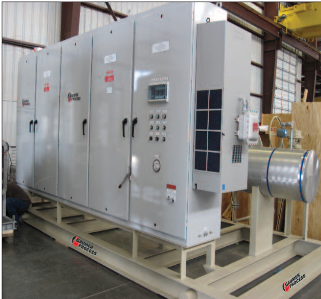
Power plant - multi-MW with air conditioning
