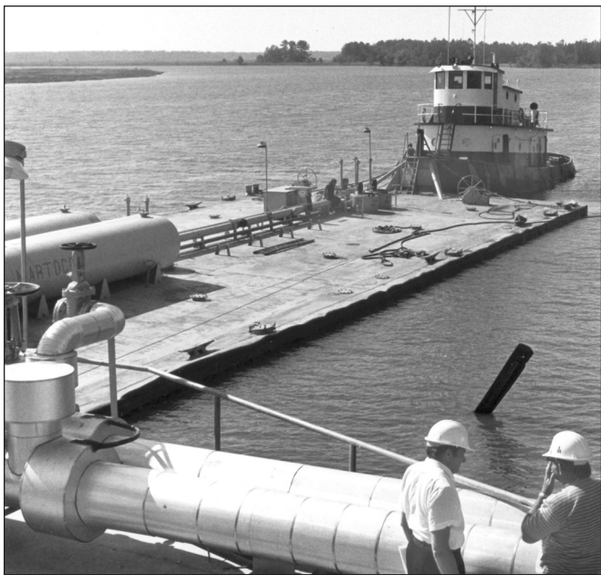
Impedance heating used to facilitate pumping of fuel oil from barges to storage tanks at power generating utility.
